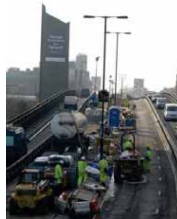
Planned (and unplanned) road and utility works completed ahead of the Games
